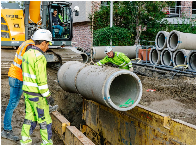
In Belgium, Tubobel builds a water system low-carbon pipes made with Betolar's Design mixes.
